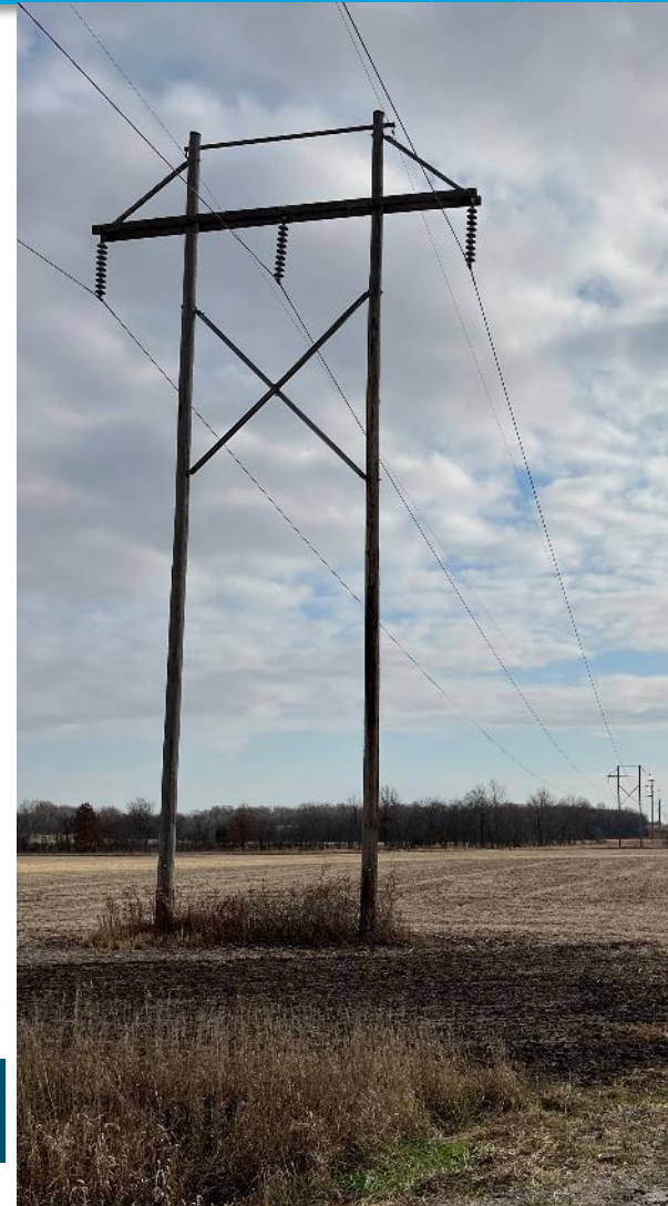
Existing 161 kV H-frame structure
