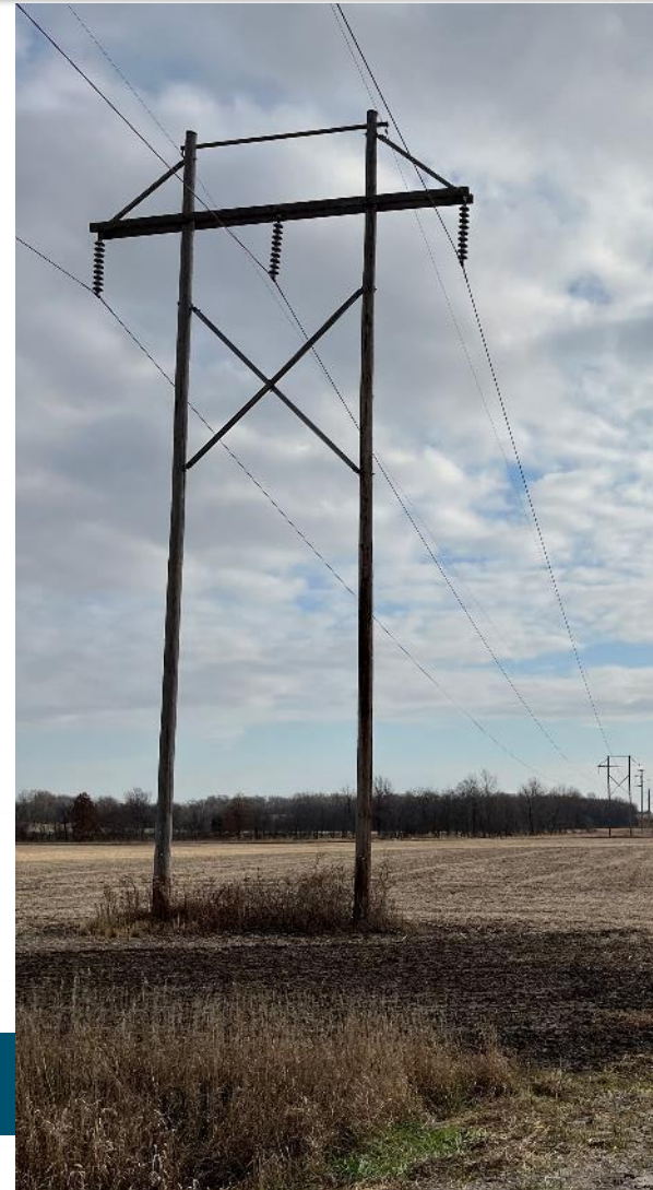
Existing 161 kV H-frame structure
