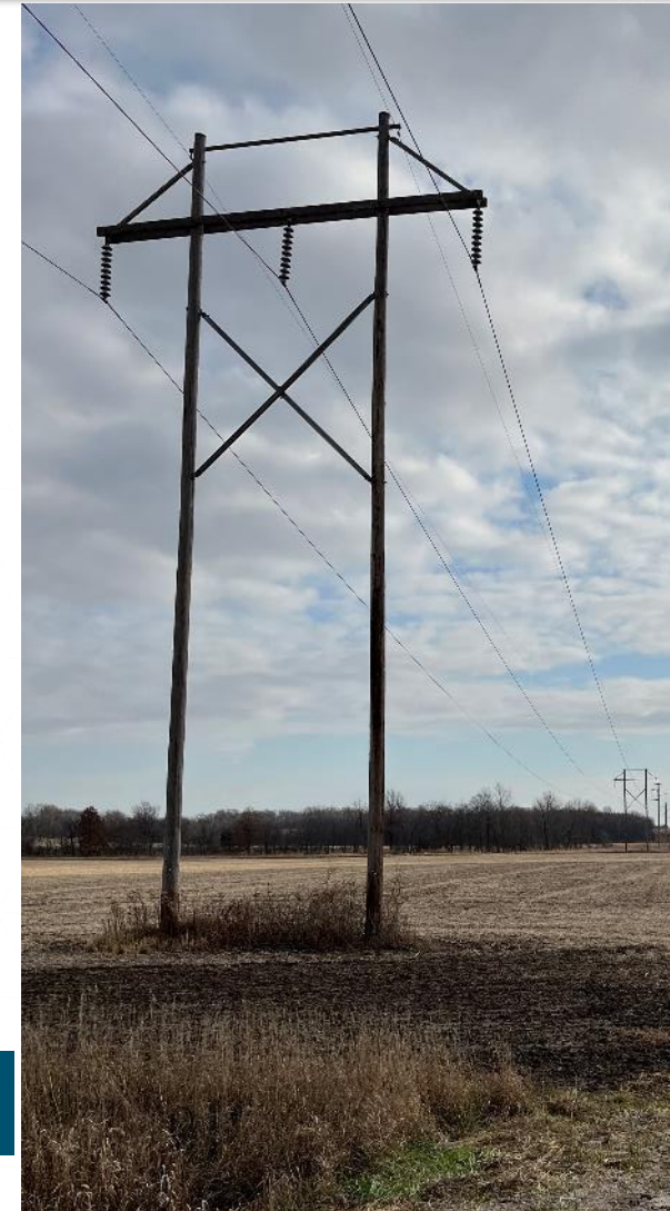
Existing 161 kV H-frame structure
